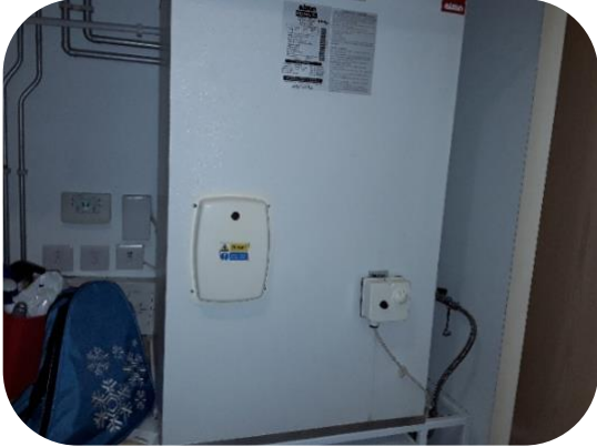
Old boiler before replacement
