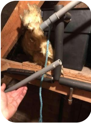
Old snapped overflow pipe
