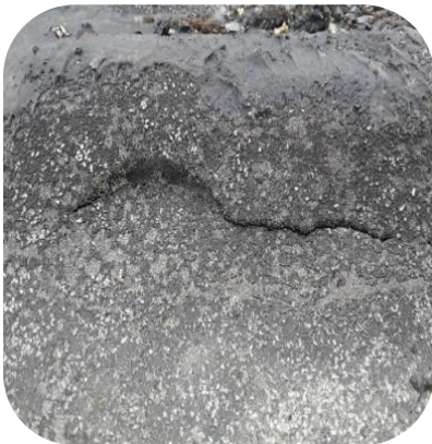
Crack on roof before repair work
