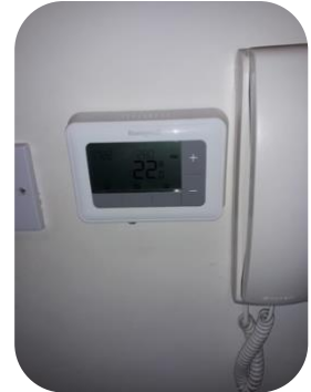
New room stat installed
