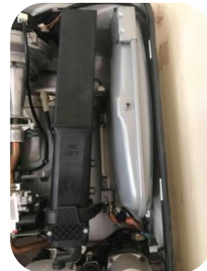
New boiler being tested during installation
