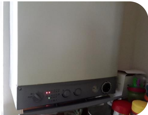
Tested boiler after re-filling system
