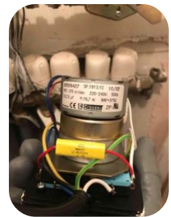
New pump motor installed
