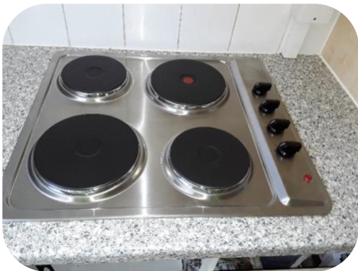
New electric hob installed
