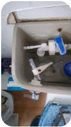
Damaged toilet handle
