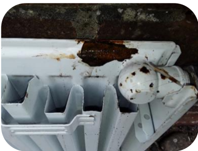
Rusty old radiator
