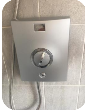
Old faulty electrical shower
