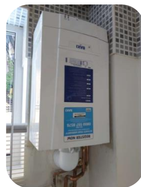
New boiler installed
