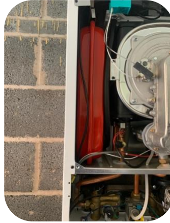
New expansion vessel installed
