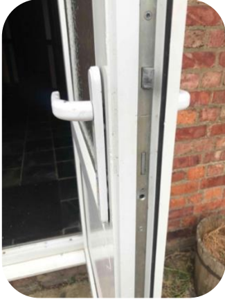
Damaged PVC door lock
