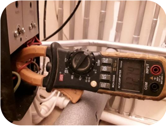
Testing boiler PCB
