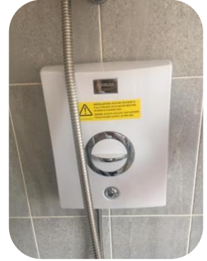
New electrical shower installed
