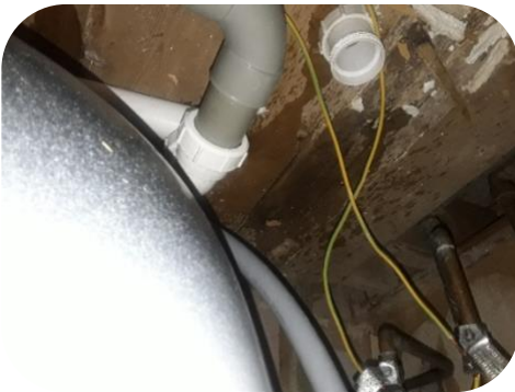
Installed bathtub waste pipes
