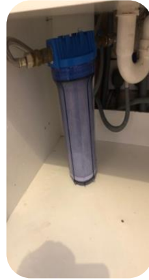
New water filter installed
