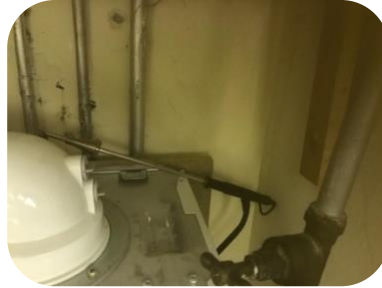
New boiler being tested
