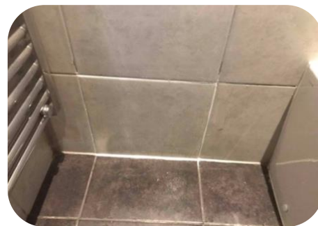
New grouts on tiles
