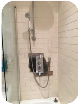
Damage caused by another contractor
