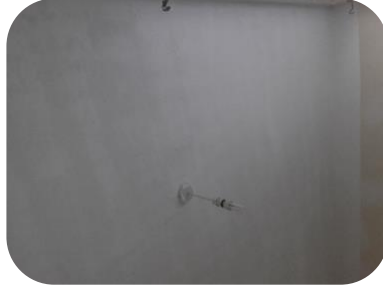
New ceiling following painting
