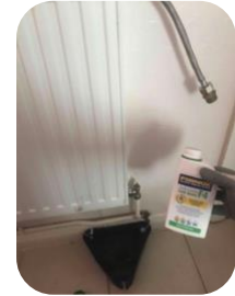
Chemicals added to central heating system
