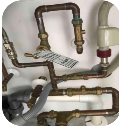
New outside stop valve
