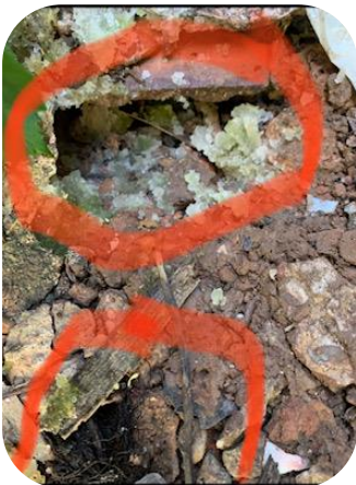
Damage in underground waste pipe system
