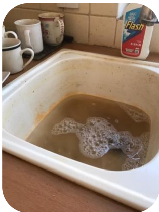
Sink blocked (before work)
